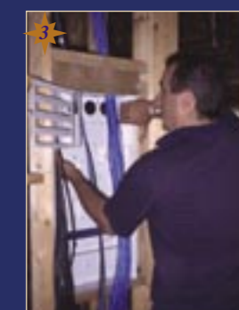
Cabinet is placed into wall ready to be screwed into its fixed position.
