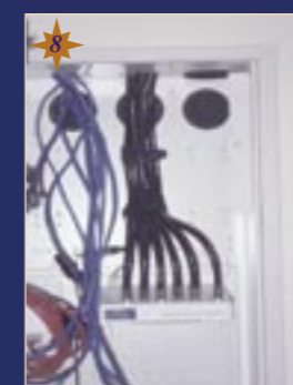
StarServe Video Hub provides whole-house distribution for Antenna and CATV signals at up to 8 television locations.
